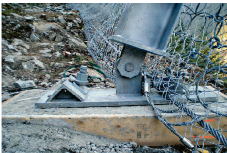
Anchorage for base plates consist of one tension anchor and one compression anchor for ease of installation. Concrete foundations are not necessary though full support of the base plate is. As such, sometimes small pads are used when in soils.
