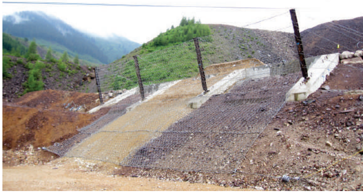
Before photo of a 3000 kJ hybrid test. The system consists of 5 m high posts with 12 m of Omega-Net.
