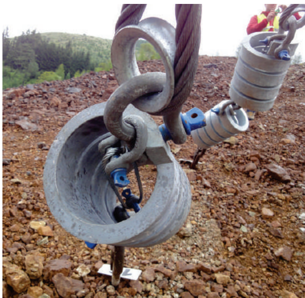
Several adaptations are made to a standard catchment fence to reduce maintenance such as the brake locks pictured above.
