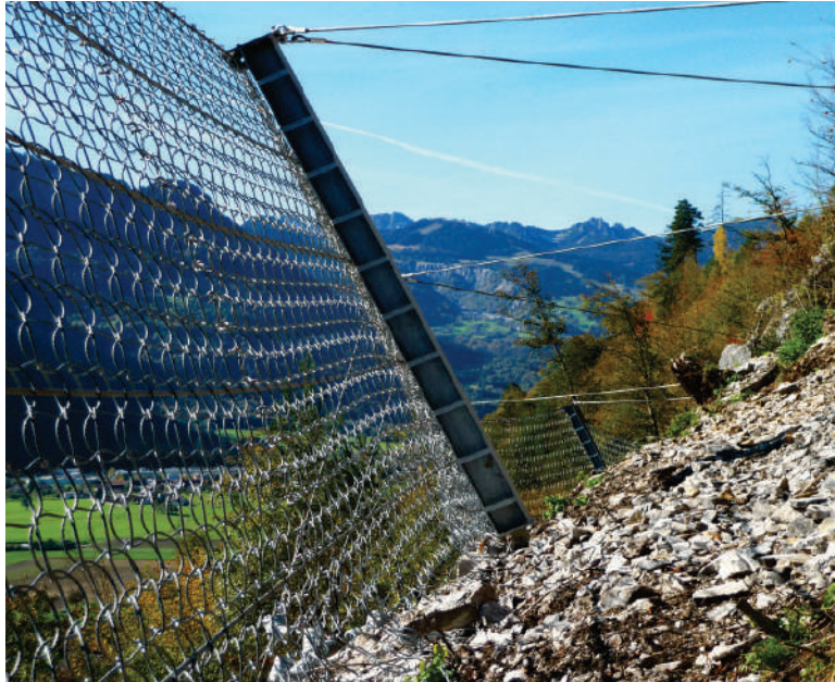
Catchment fences with a hinged connection between the post and base plate require upslope anchors and retaining ropes. As such, large energies can be accommodated while minimizing forces on the foundation of the post.
