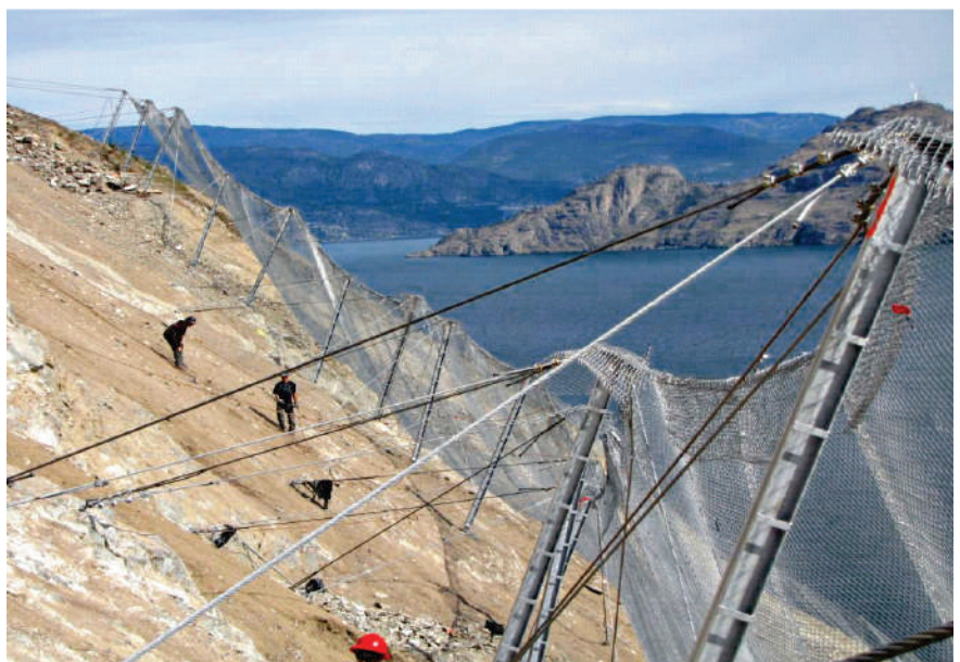
A lower energy attenuator system composed of High Performance Netting in combination with standard hinged posts and base plates.
